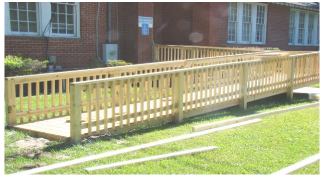
ADA ramp at Appling County is built with AARA quality improvement funds.
